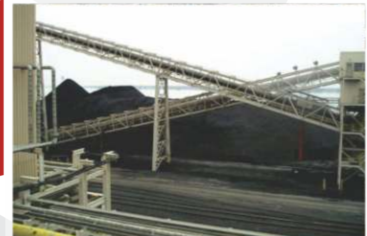
Coal Handling System
