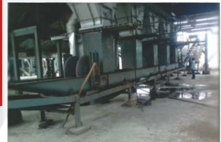
Ash Handling System
