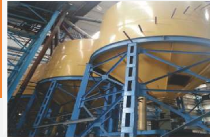
Sugar Silo System With Auto Weighing And Conveying System
