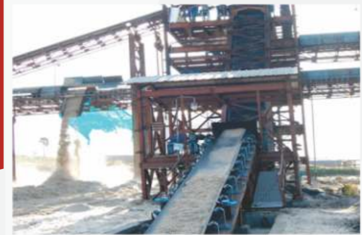
Bagasse Handling System
